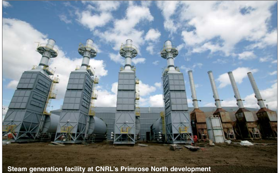
Steam generation facility at CNRL's Primrose North development
